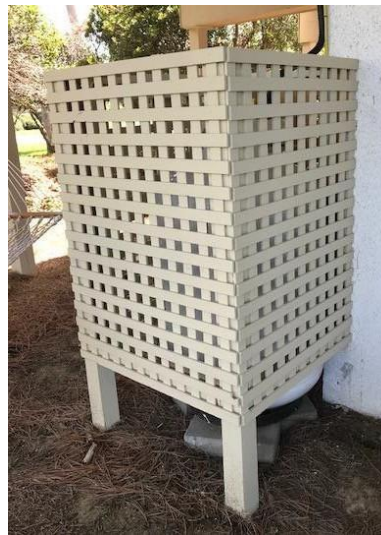
Figure 7b Propane Tank Enclosure (right side)
