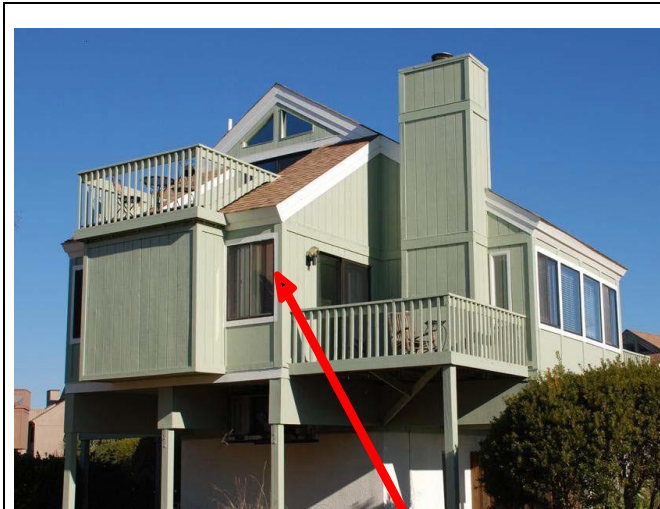
Figure B-4 Master Bedroom Window with Non-standard Trim Width Showing “Simulated Trim”
