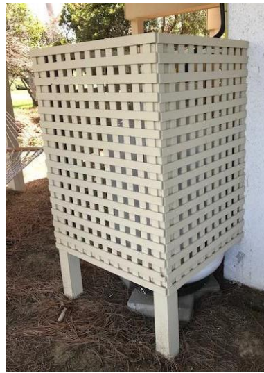
Figure 7b Propane Tank Enclosure (right side)
